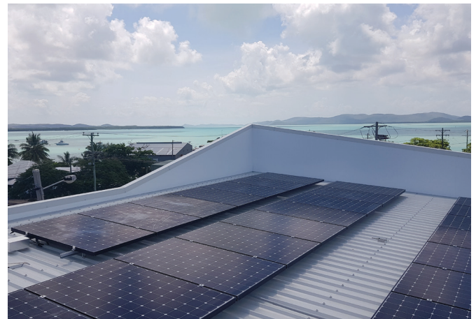
Figure 19 – TSRA 70kW Rooftop Solar PV System, Thursday Island. Photo courtesy of TSRA.
