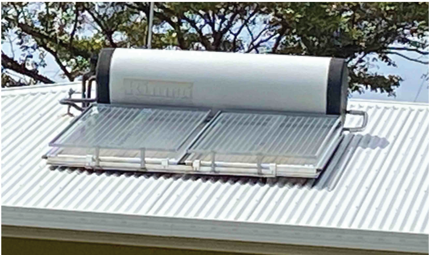
Rooftop Solar Hot Water System
